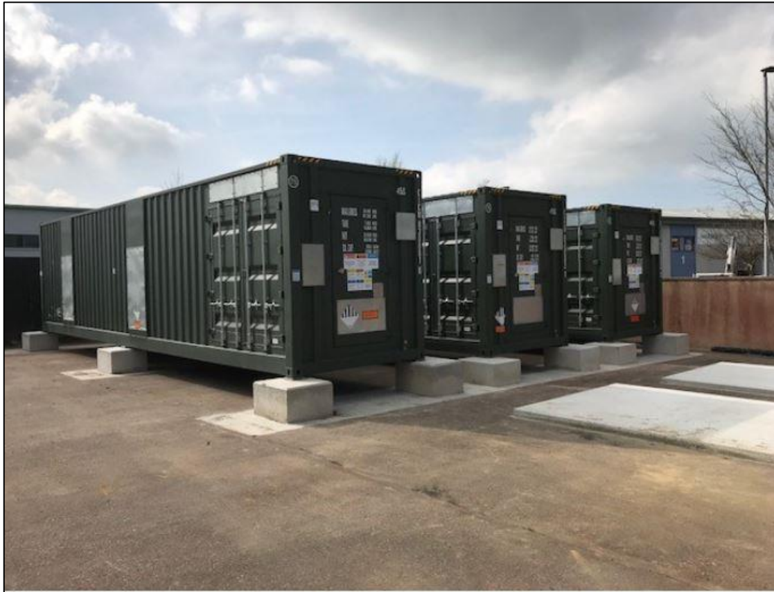
Figure 2: Example Raised Container Units 7
