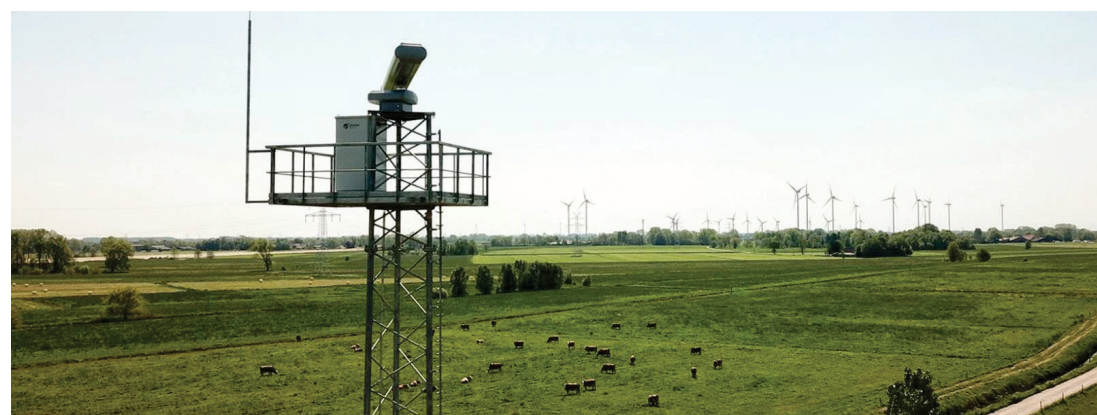
Figure 10 Terma 5002 Radar at a Wind Farm in Germany
