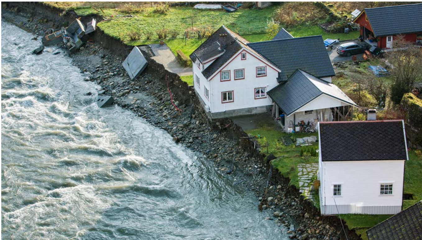
Extreme weather has major consequences. Pictured here from Flåm in Norway where heavy rainfall made the river overflow its banks, causing severe damage. Photo: Tore Meek/NTB scanpix.
