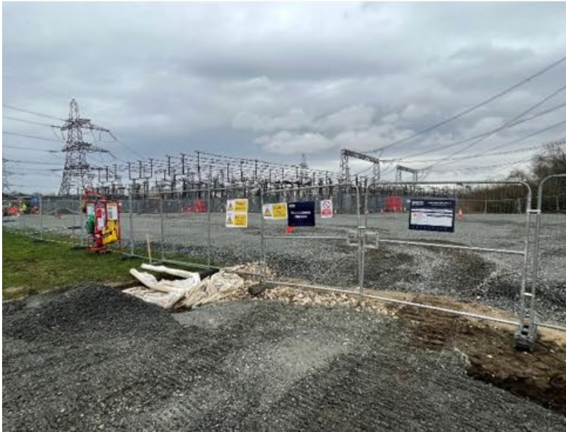
400kV CDM Area – post handover
