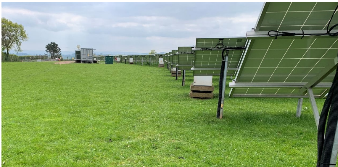
Photograph 22: Example of Land Above Buried Cables, Monmouthshire
