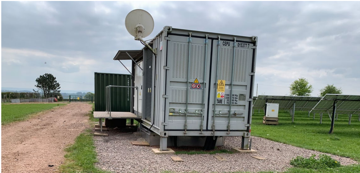
Photograph 26: Typical Inverter Containers
