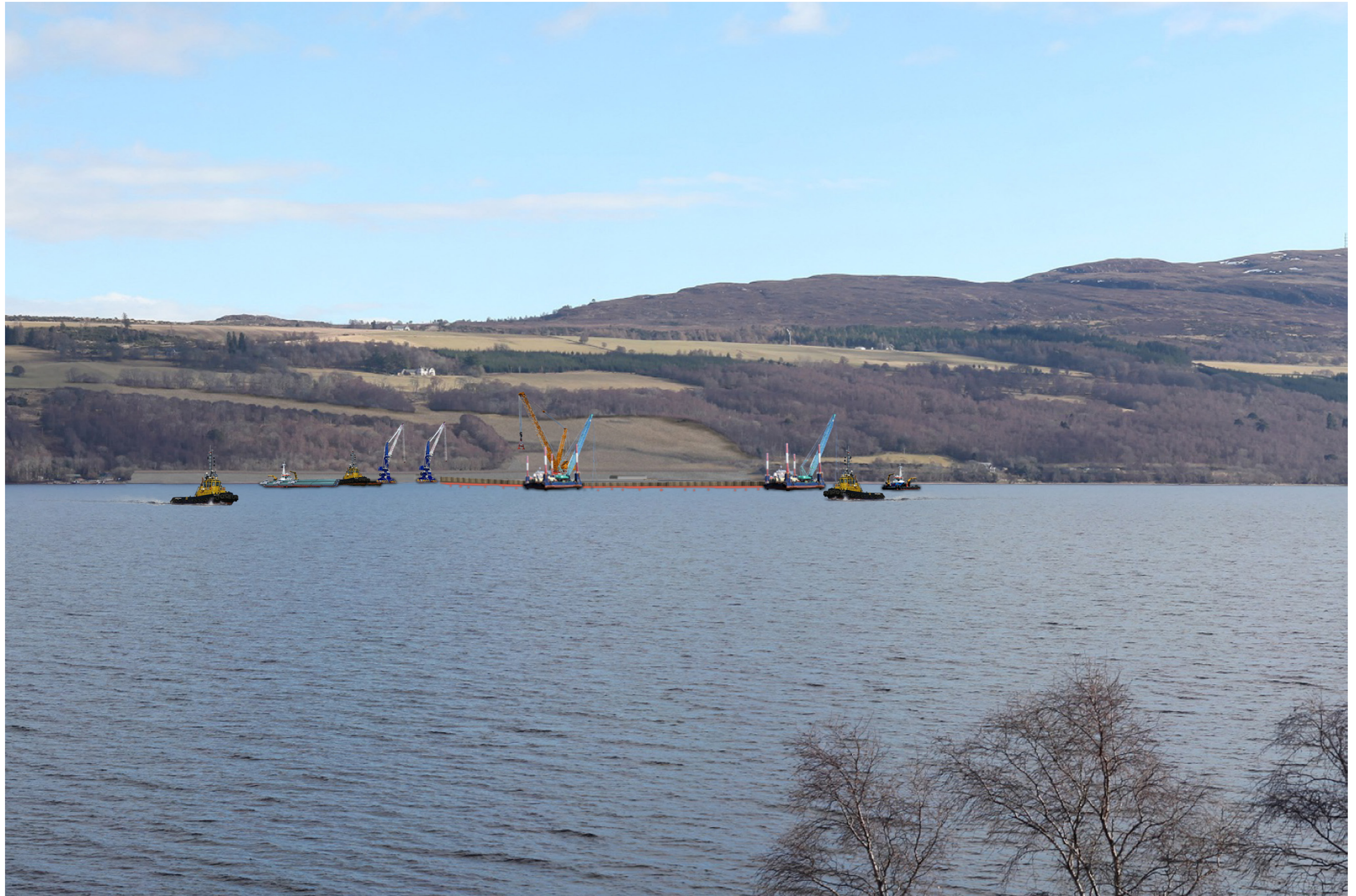
Viewpoint 10 -Layby on A82 Photomontage during construction, Year 2, Tailpond construction, 75mm Focal Length
