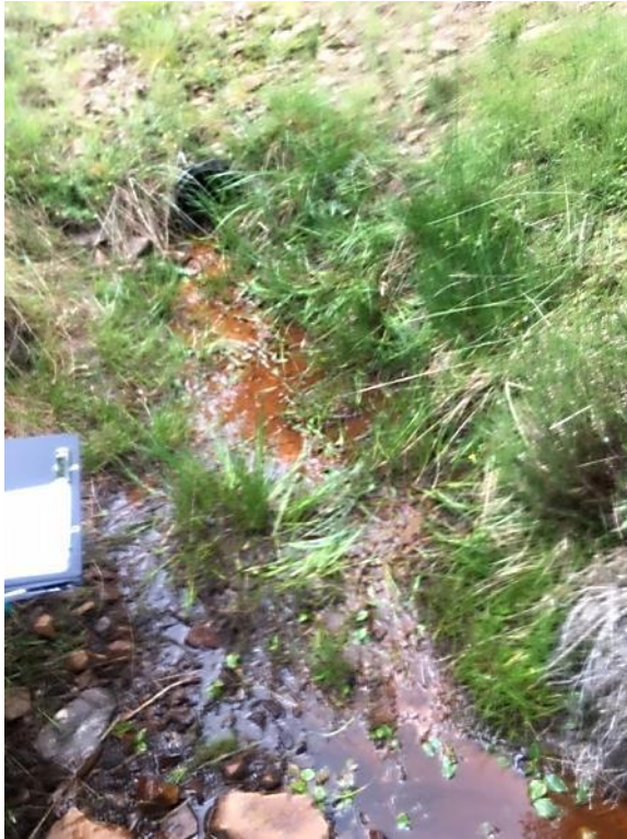
Plate 7: Outfall pipe present at site KS06 with potential water contamination of ochre.
