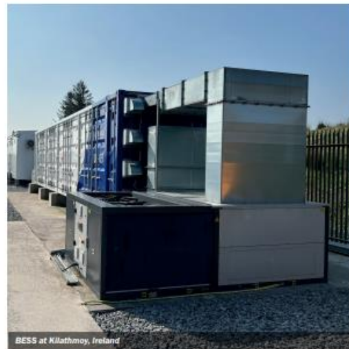
BESS at Kilathmoy, Ireland
